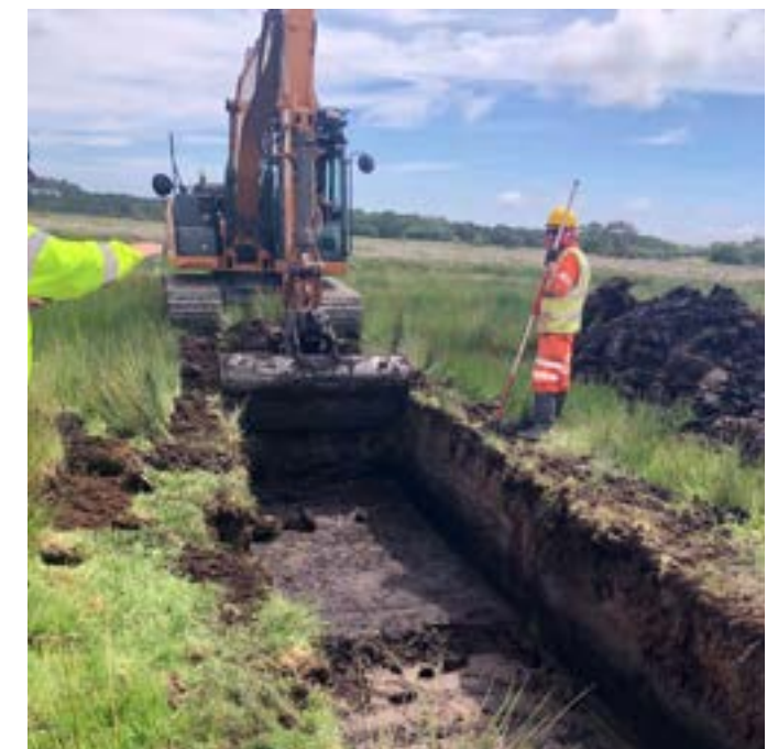
An excavator digging a trench with an archaeologist looking for artefacts and soils information.
